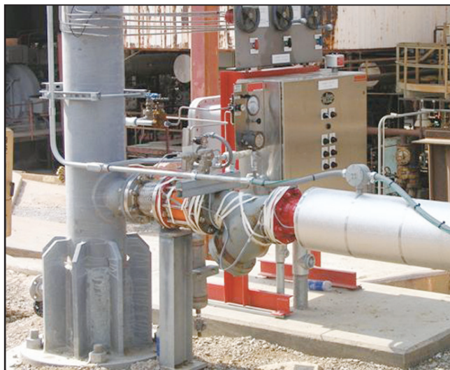
Control panels located throughout the system provide operations and emergency instant on capabilities
